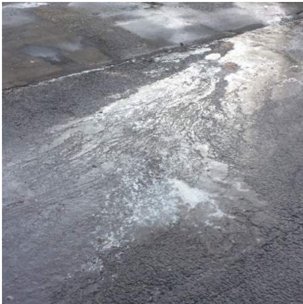
Figure 13: Larger hardstandings with poor drainage can cause flooding; in this example cold conditions led to the road being iced over (source: HWNPF)
