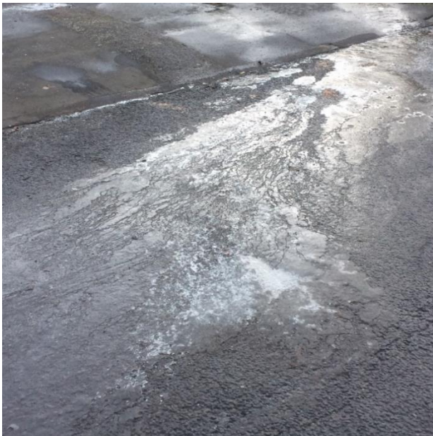
Figure 13: Larger hardstandings with poor drainage can cause flooding; in this example cold conditions led to the road being iced over.
