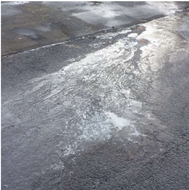
Figure 13: Larger hardstandings with poor drainage can cause flooding; in this example cold conditions led to the road being iced over (source: HWNPF)
